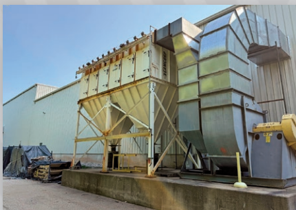
100 HP Camcorp Dust Collector
